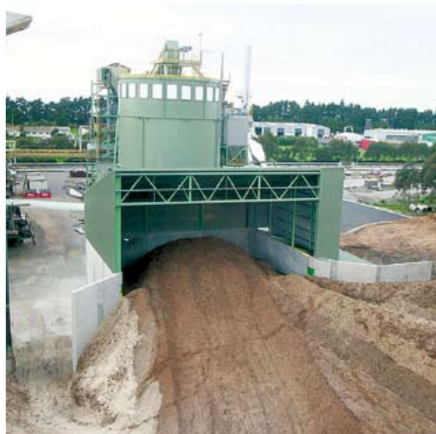
600m 3 Pull Floor Reception Bunker
