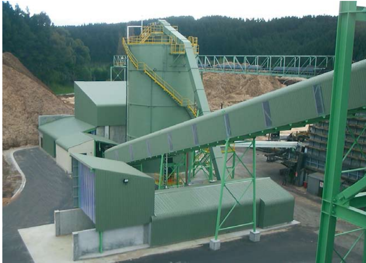
Pan Pac Forest Products. Shaving reception (front), 800m 3 shavings silo, 600m 3 pull floor bunker (rear)
