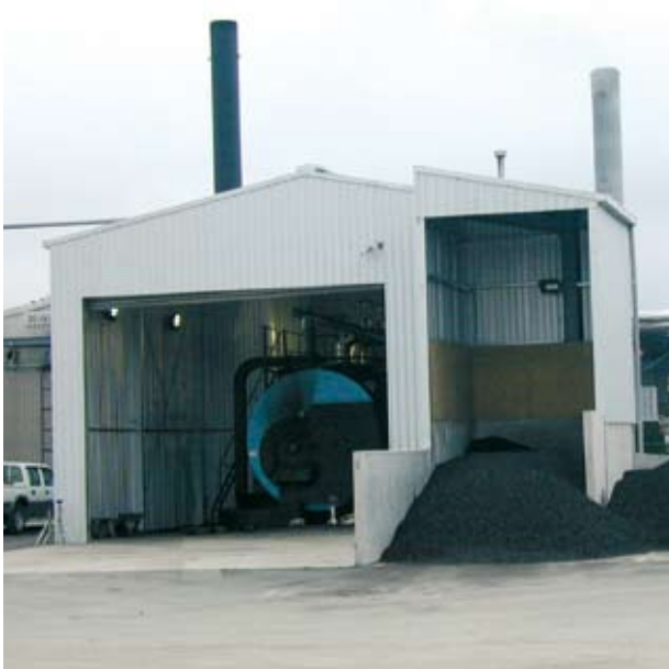
KLC Coal Reception Storage and Feed System
