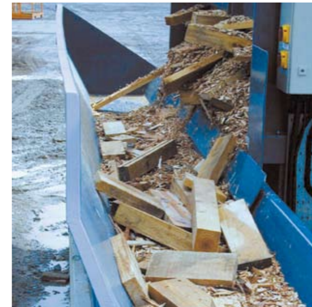
Discharge conveyor unscrambled product
