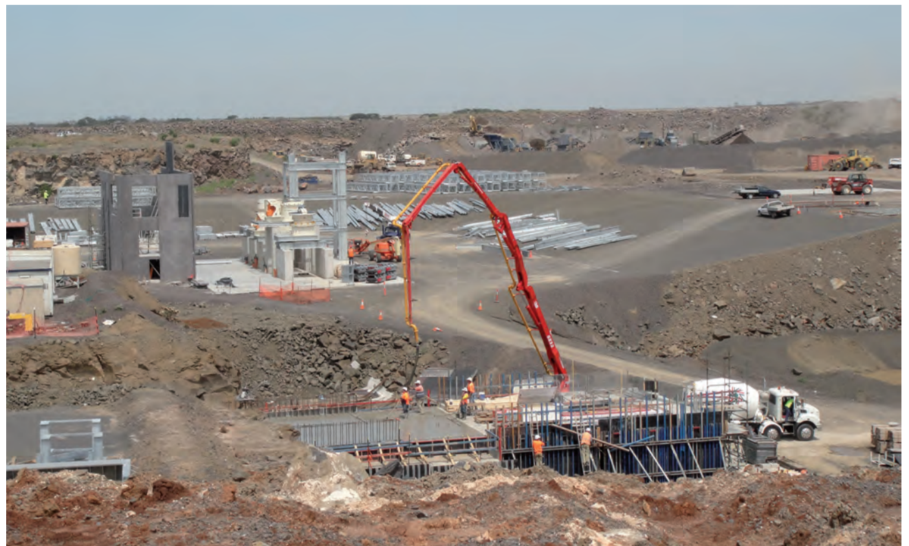
The Wyndhamvale Quarry. Foreground: The primary station; Background the secondary and tertiary crushing buildings
