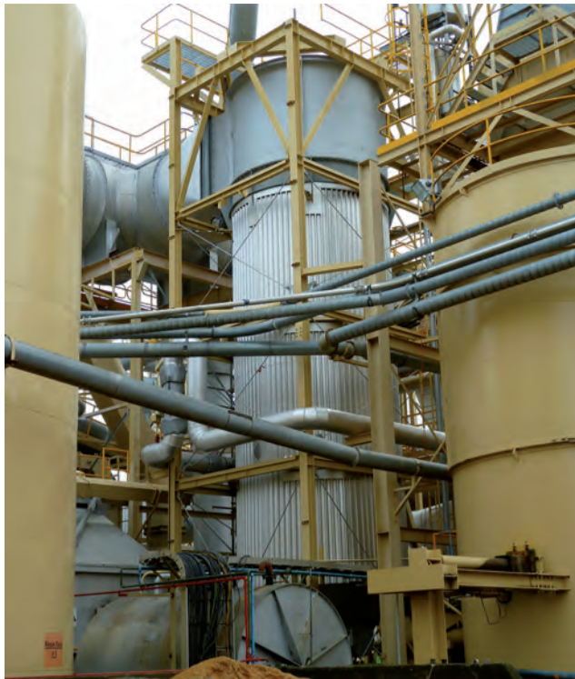
Installed and operating Heat Exchanger
