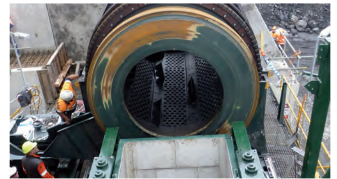
Photograph shows the final positioning of the Rotary Breaker and the new Screen Underpan (foreground)
