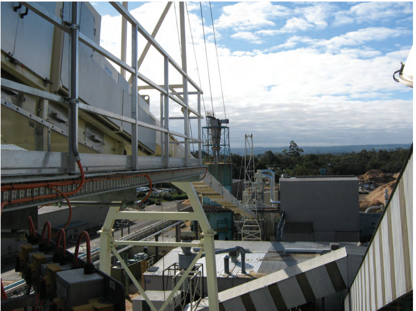
View from Receiving Silo Back Along Tubulator to PZK Building
