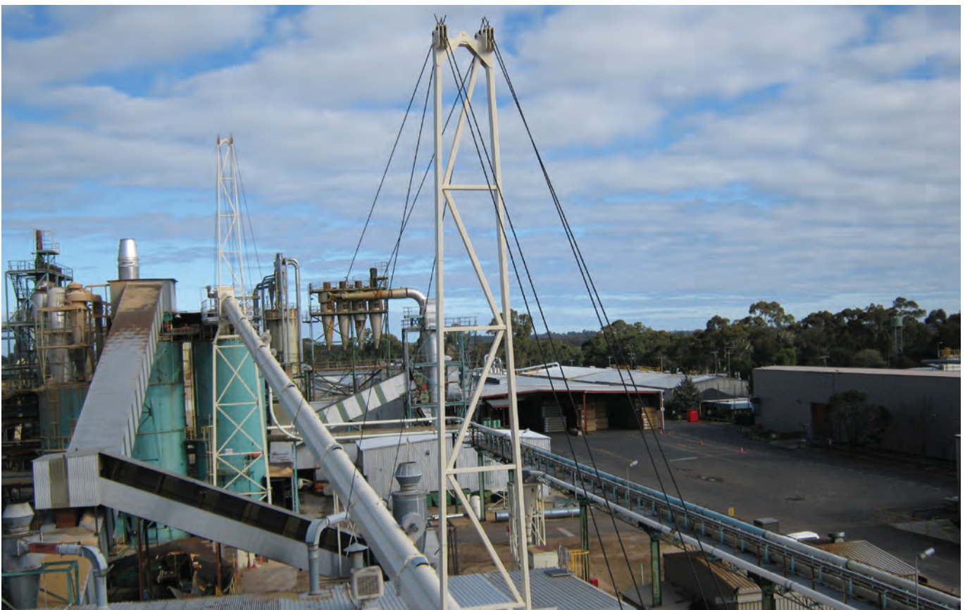
Completed Installation (Feed View)
