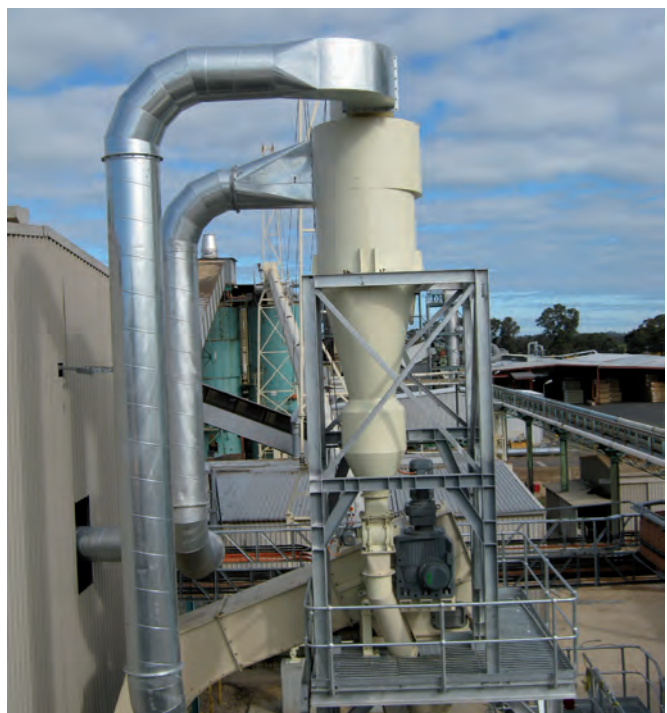
Completed Aspiration System & Transfer Tower
