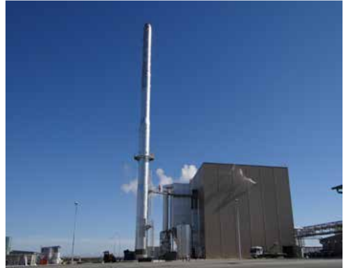
Boiler Stack installed in North Otago
